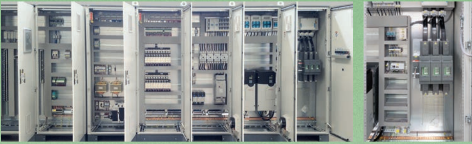
TRATTAMENTO ACQUE - Water Treatment
